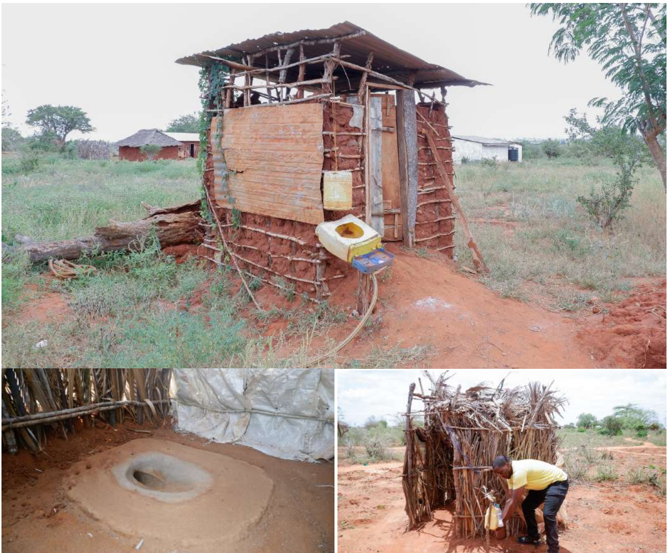
Samples of low cost latrines constructed by community members through the CHEPs CLTS program
