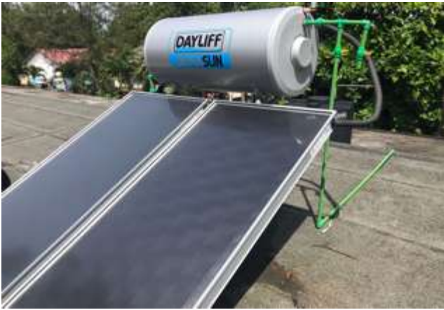
Hot water solar system installed
