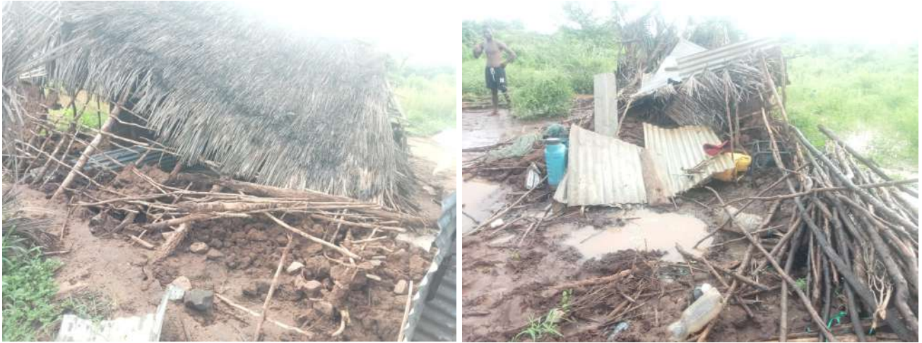
Some homes that were destroyed by floods
