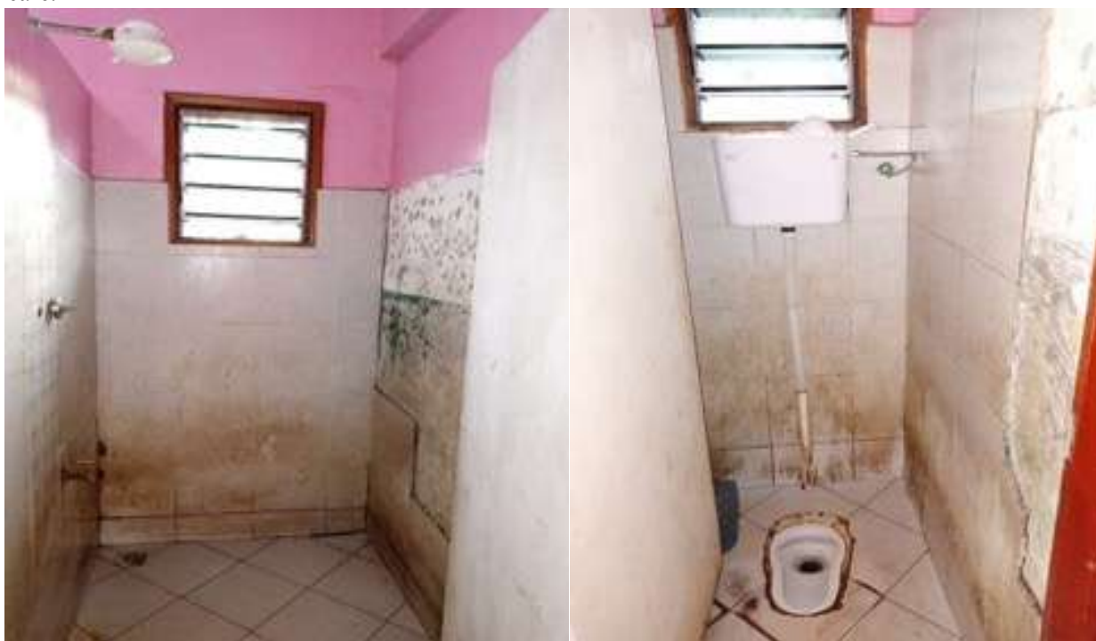
Previously dirty toilets
